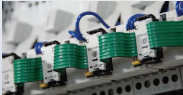
Figure 1. Recent innovations in control panel wiring methods can reduce the costs of manufacturing and ownership.
