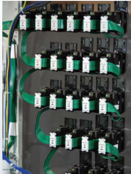
Figure 6. Device-level wiring systems use flat multiconductor cables to connect components, replacing bulky wiring ducts found in conventionally wired control panels.
