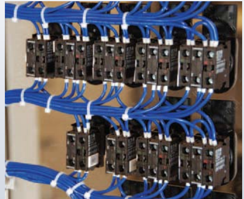
Figure 2. Additional control panel construction time is required when wiring is bundled to door-mounted devices because wires must not restrict opening and closing the door.
