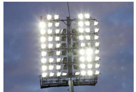
Stadium / Street Road lighting
