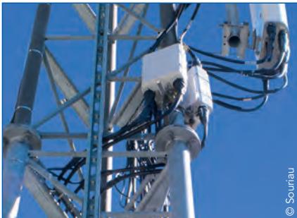
Cell Tower Distribution Box
