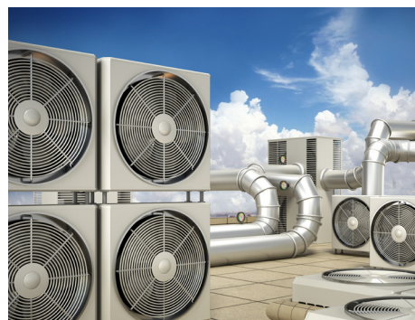
Rooftop AC System
