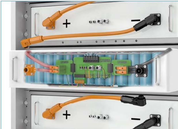
View inside a storage module with battery packs, balancing printed circuit boards, and both internal and external interfaces.
