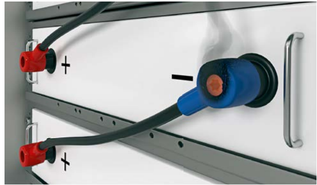
Screw connections for power transmission harbor the risk of large temperature increases due to increased contact resistance.
