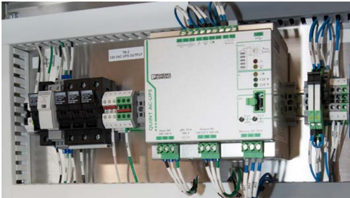
Figure 3: Because the Class CC fuses are Class I, Division 2-approved, Xenon does not have to purge the panel.
