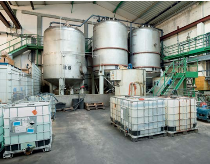
Figure 2: Tanks for separating the emulsions delivered.
