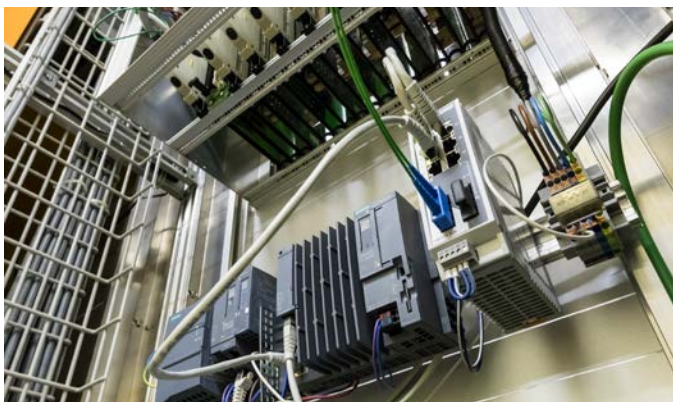
Fig. 2 The control technology installed in the substation is connected to the fiberglass ring via the FL Switch 2206-2FX-SM.
