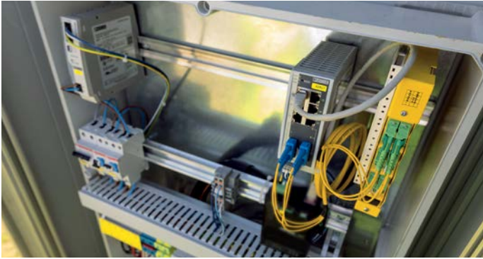
Fig. 4 The 2000 series switch is also used to couple the sign gantry with prism rerouting signs to the fiberglass network.
