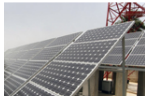
Solar-Powered Cellular Base Station
