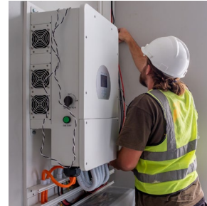
Energy Storage Systems
