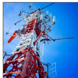
Telecommunication Base Station
