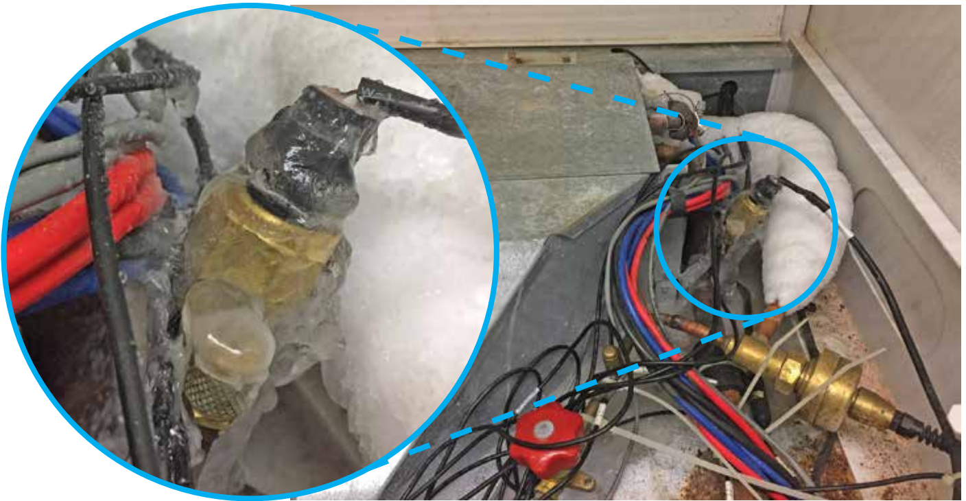
Figure 1. PX3 Series in Actual Industrial Refrigeration Application
