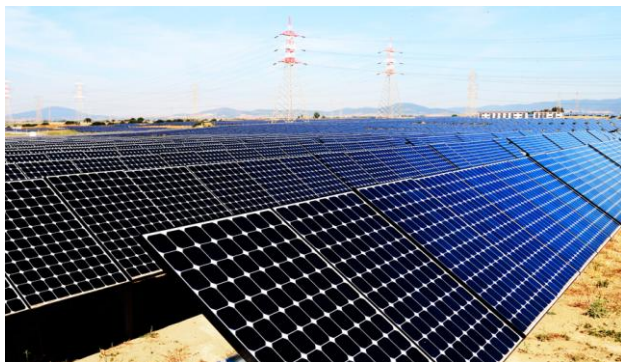
Figure 17. Ground-Based Solar Panels
