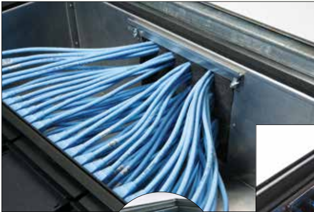
Firestop block adds protection to network wiring.
