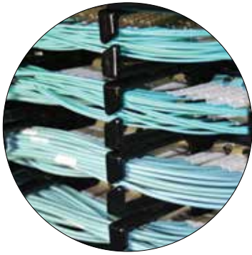
Front cable management
