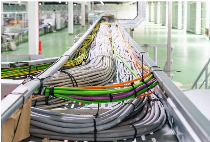
Figure 2: High-speed wired communications on the factory floor
