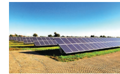
Solar and Inverters
