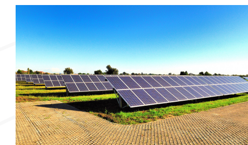
Solar and Inverters
