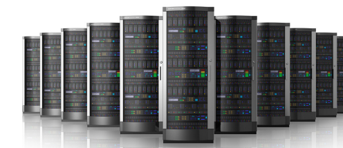
Communications and Data Center
