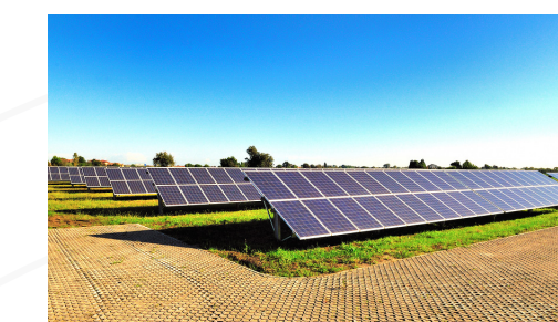
Solar and Inverters
