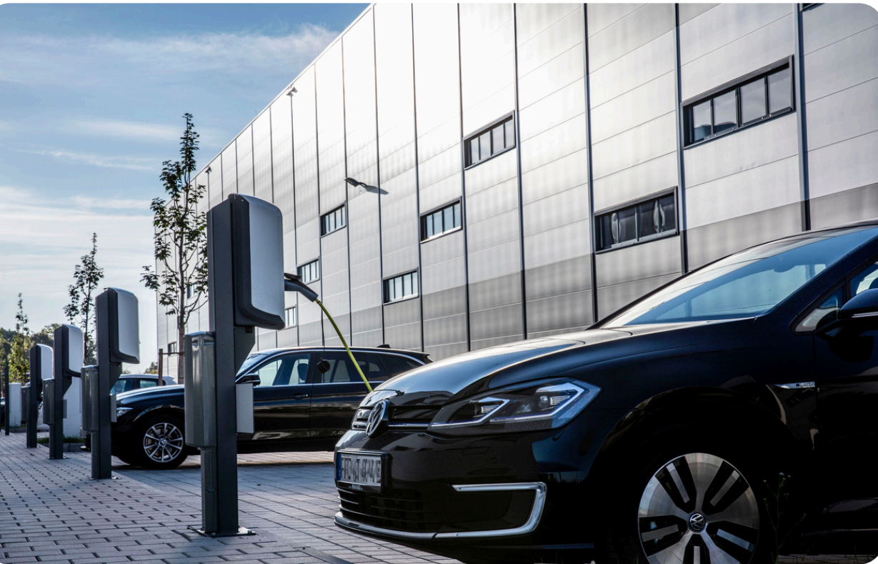
EV charging station powered by rooftop solar at our Maisach, Germany location
