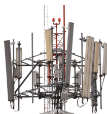
Remote Radio Units (RRU)
