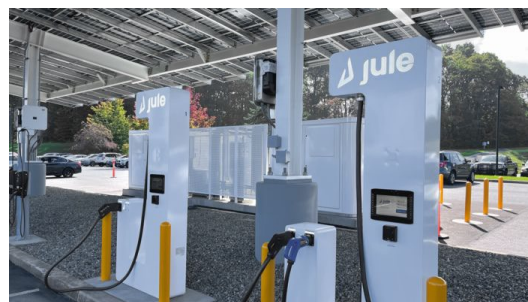
4 E-mobility charging park, USA
