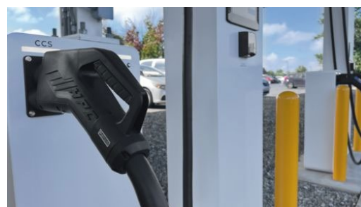
3 CCS1 charging station, USA
