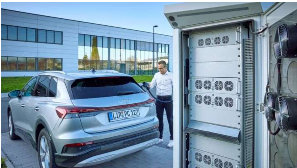
Figure 3: DC charging at building 60 in Blomberg
