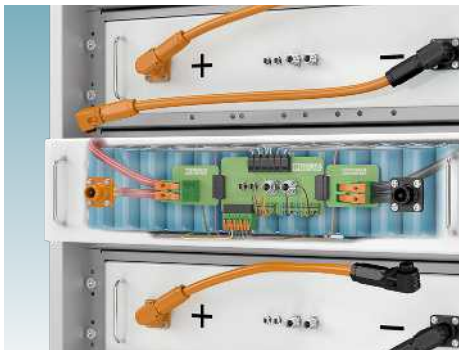
Battery management systems
