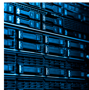
Data Center Server
