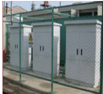
Large-scale Power Storage
