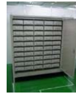
Mid-range Power Storage
