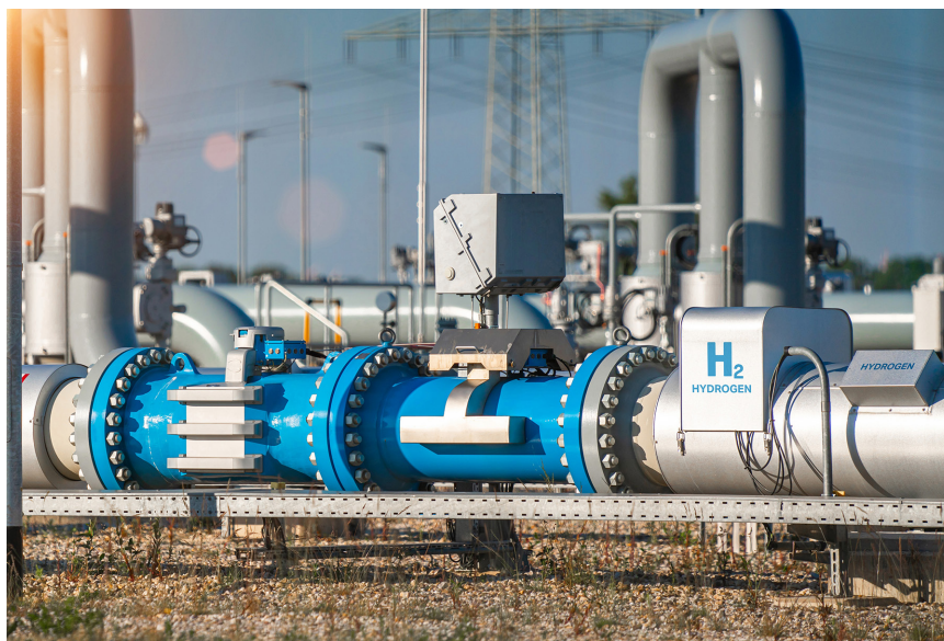
Figure 5. Hydrogen Storage Facility and Pipeline Network
